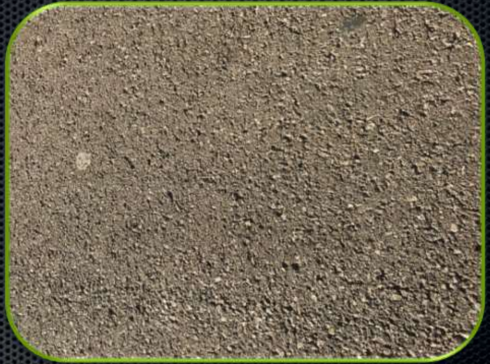
Early Pitting of asphalt
