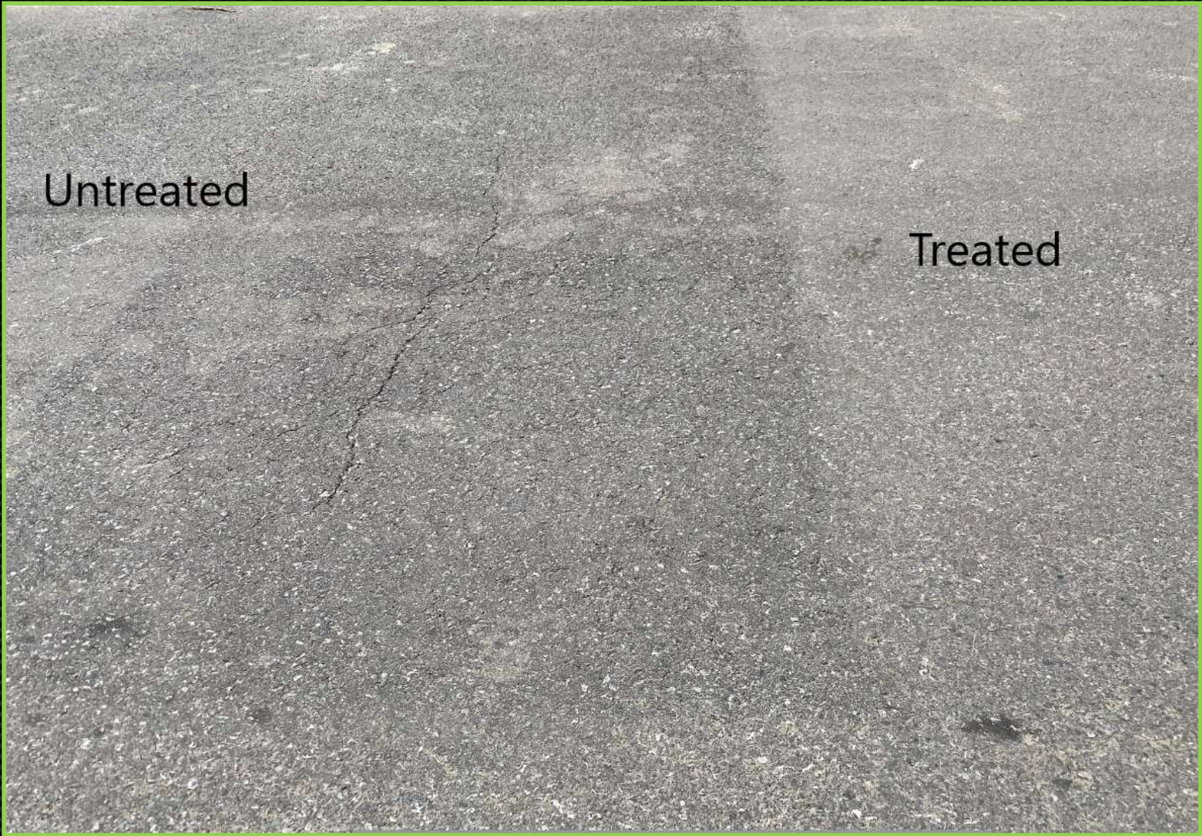
Closer look reveals slight surface cracking in untreated area vs treated section. Pitting is also more evident.
